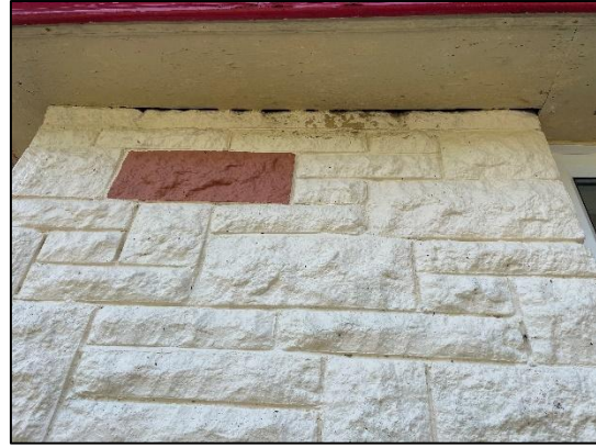
Plate 4-2 External entry point with bat droppings on the wall
