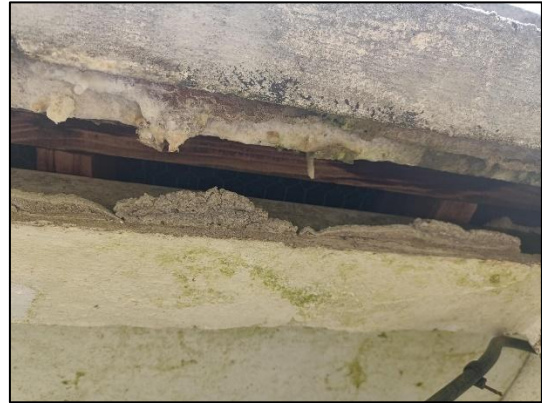
Plate 4-19 Large cavity in flat roof section of outbuilding
