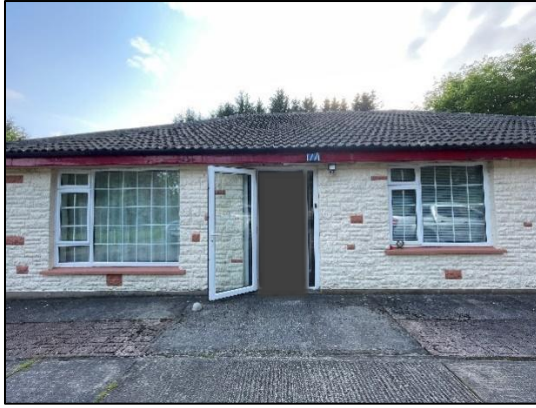
Plate 4-1 Derelict dwelling with a confirmed roost
