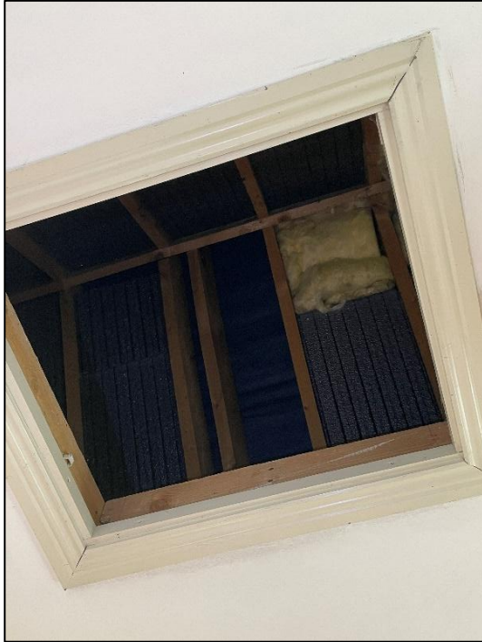
Plate 4-7 Fiber glass insulation
