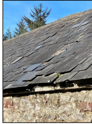
Plate 4-12 Entry point - Loose slates
